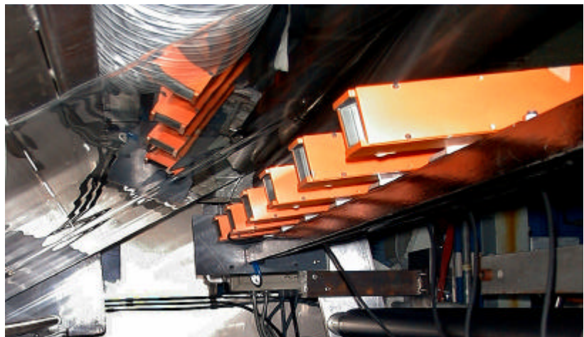
Micro profile monitor installed on a film processing line
